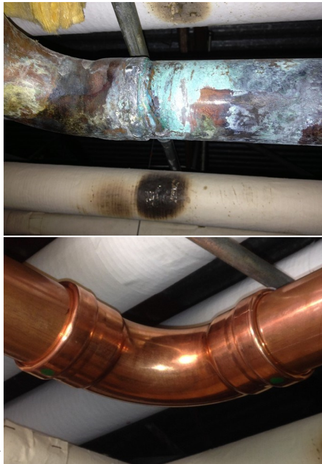
Image 1—Before and after corrosion of main water pipe in East Tennessee Regional Health, Knoxville
